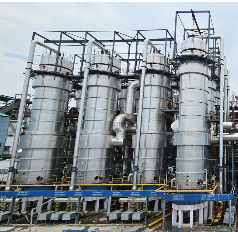
6 Nos. 5500 m 2 & 3 Nos. 4500 m 2 HSA FFE at DCM Shriram Ltd. (Loni Unit) U.P, India
