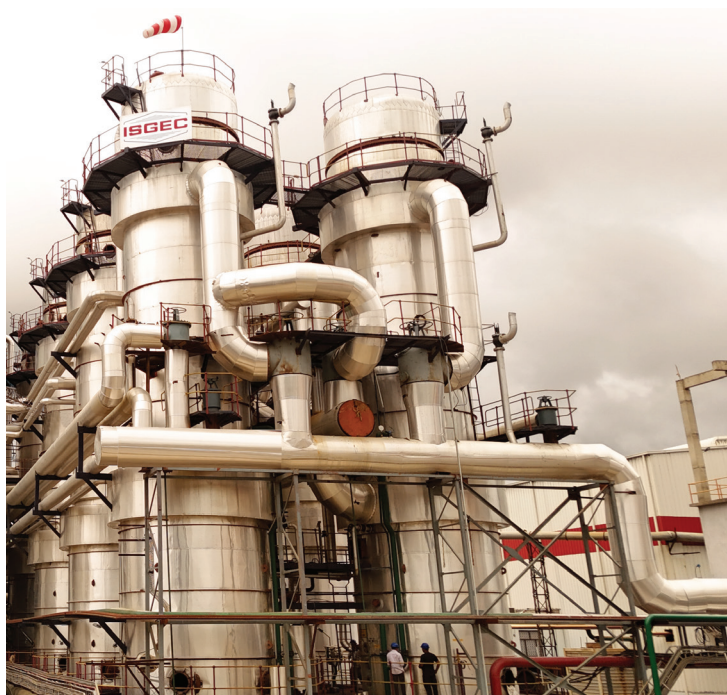
8 Nos. 5000 m 2 & 2 Nos. 2000m 2 HSA FFE at Bindal Paper Mills Ltd., U.P, India
